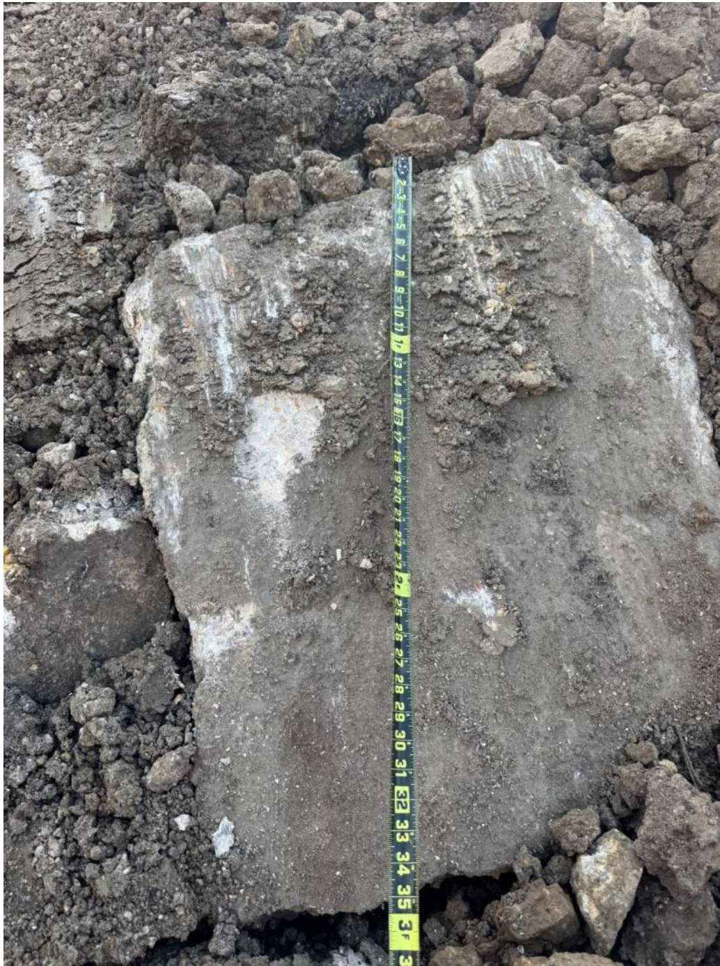
Photograph 4: Concrete rubble in sidewall in east edge roughly 4 feet up from toe of slope
