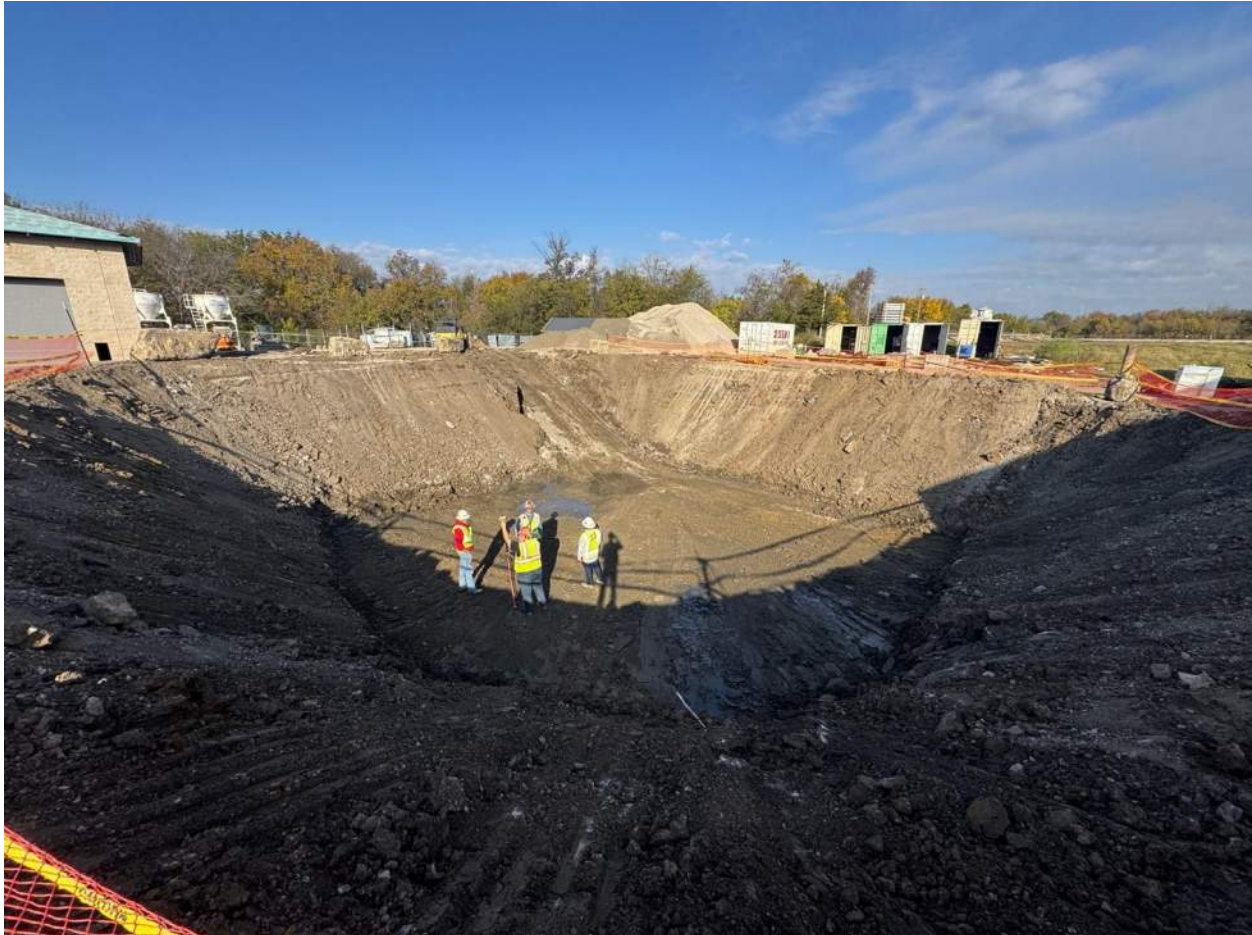
Photograph 1: Observed excavation at time of visit
