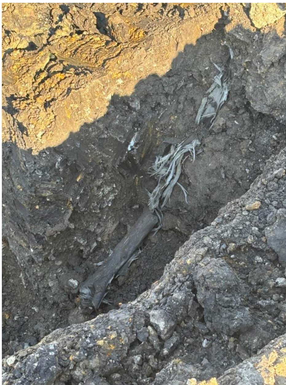
Photograph 9: Timber buried within test pit excavation
