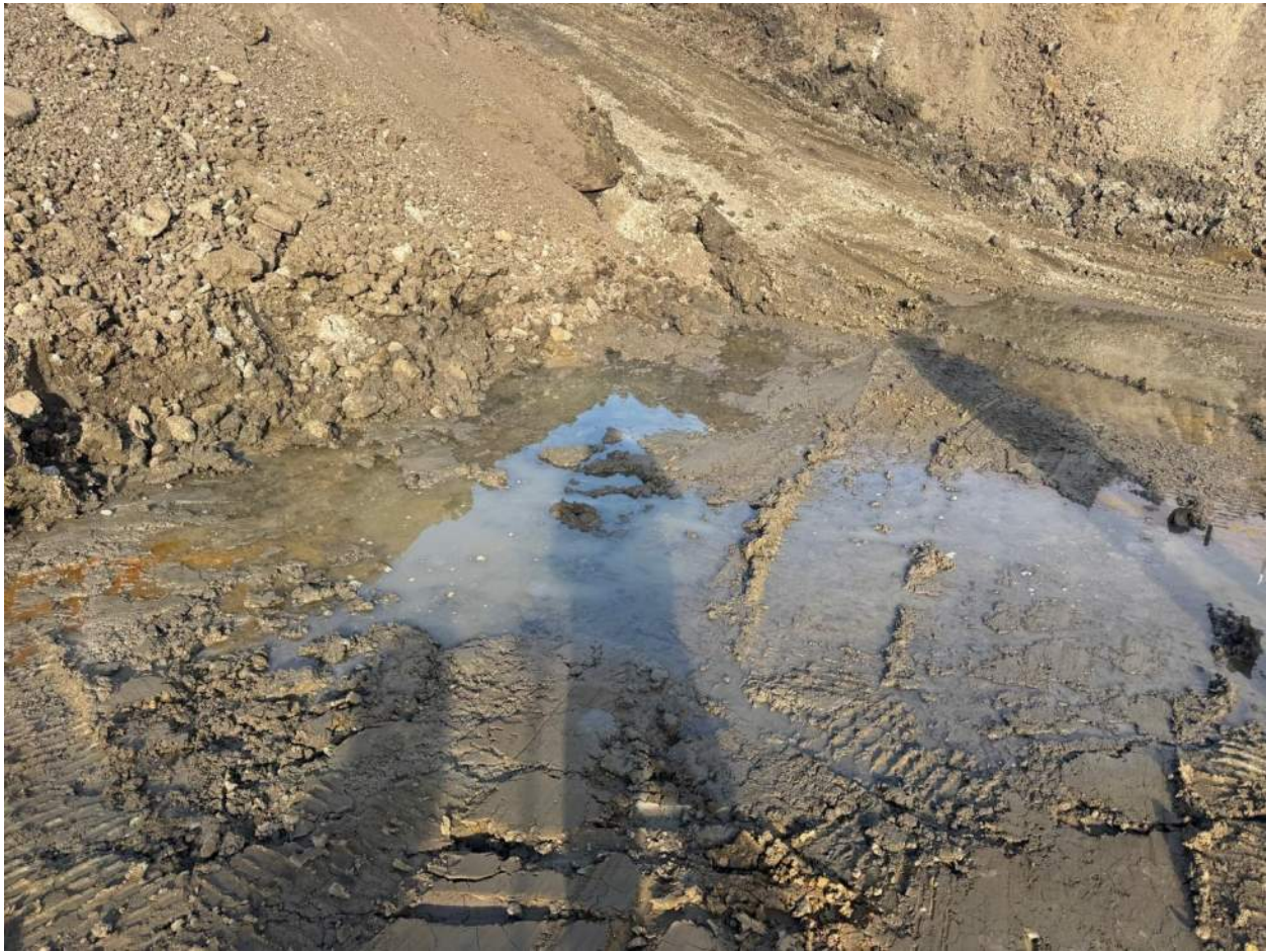
Photograph 2: Standing water in west edge of excavation less than 3 inches in depth
