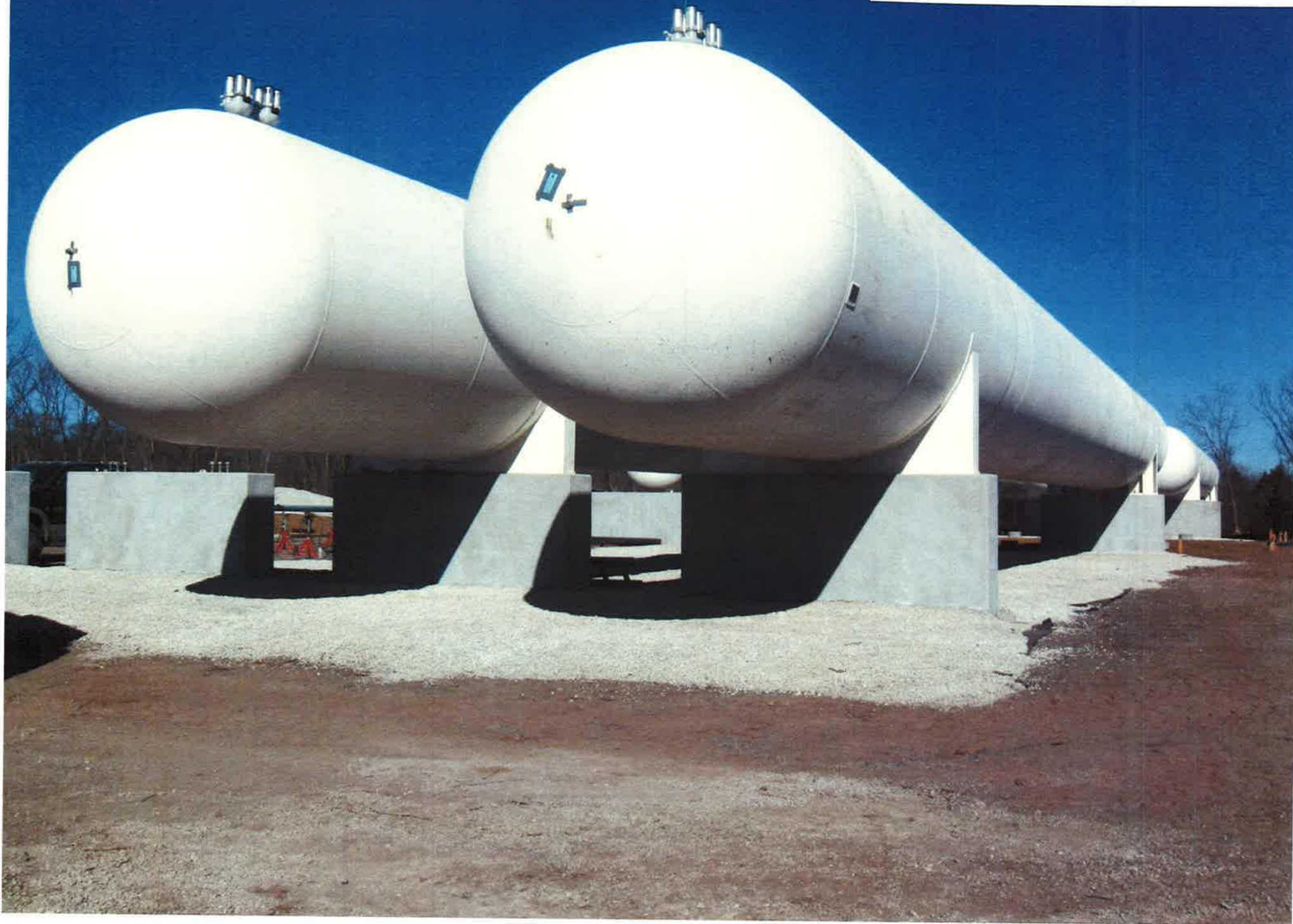
TEXON Petroleum Blending Facility
