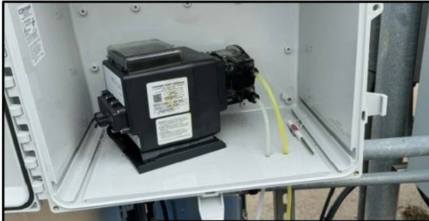
Scent abatement pump and barrel installed at Newman Lift Station
