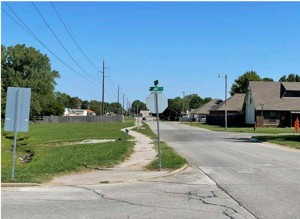
Existing Asphalt sidewalk, with fading crosswalk striping. N. Warrior Road from 144 th Pl.
