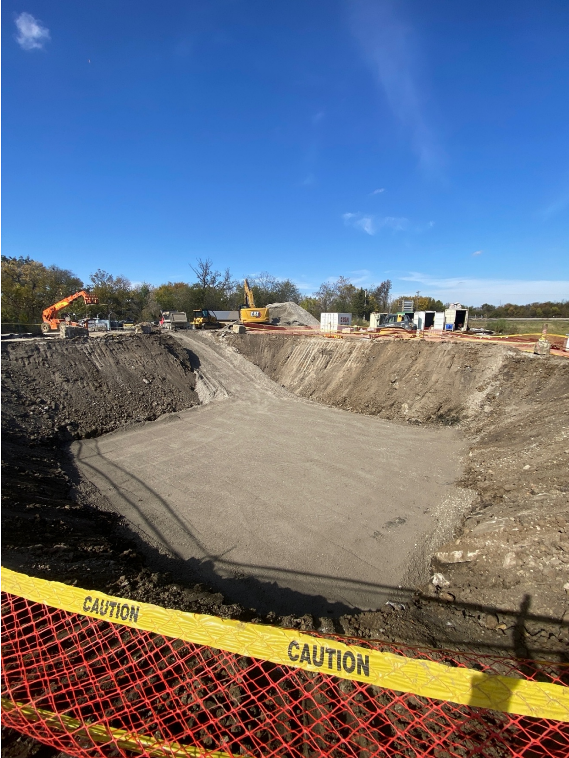
Solid Dewatering Facility
