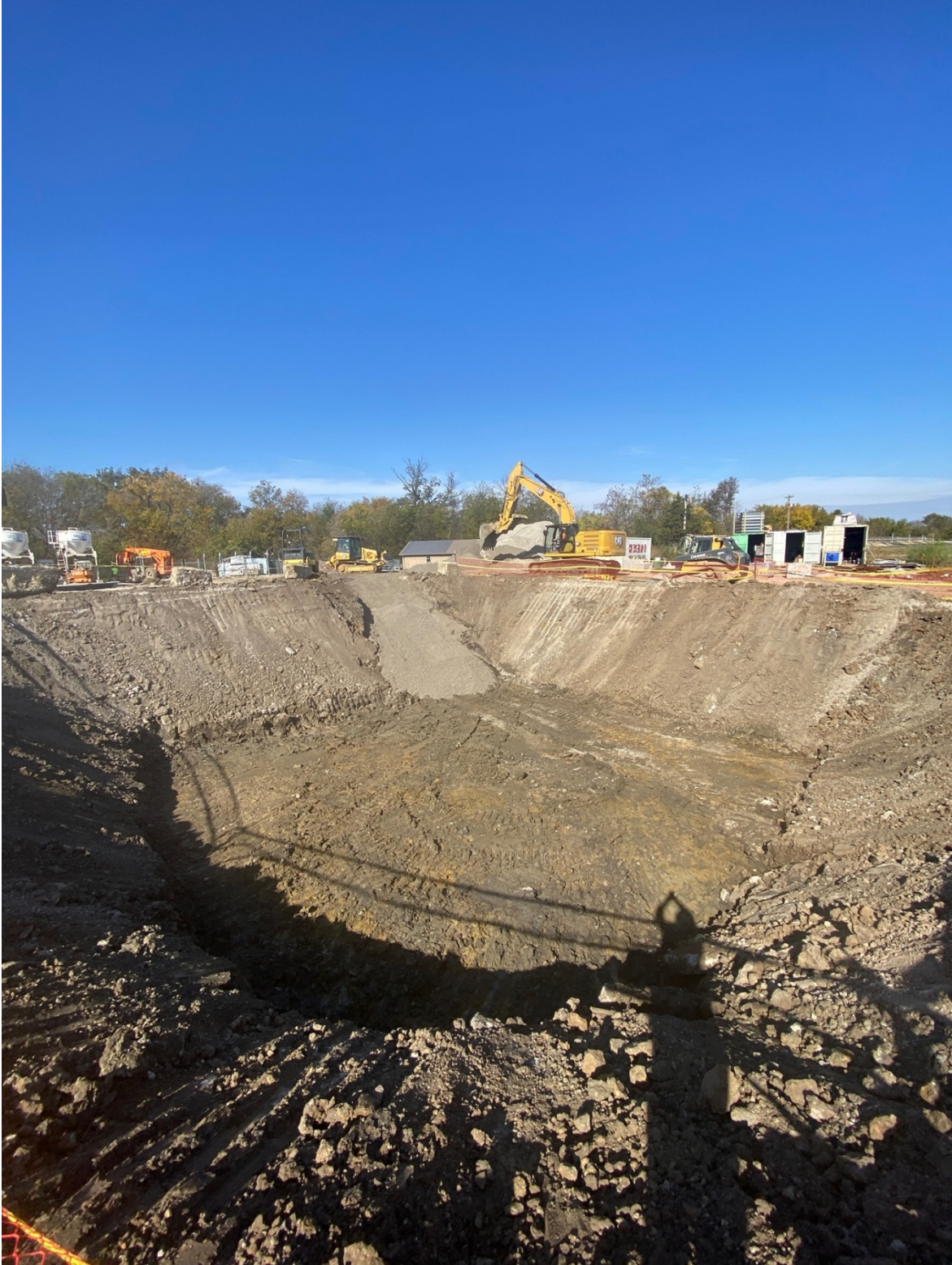
Solid Dewatering Facility
