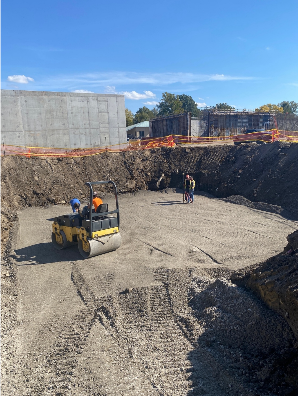
Solid Dewatering Facility
