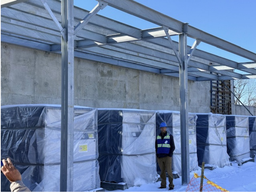
7 BLOWERS DELIVERED FOR THE SBR TANKS AND DIGESTERS
