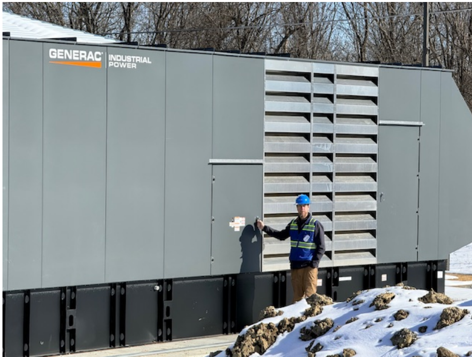
1 MEGA WATTS'S GENERATOR FOR THE WWTP
